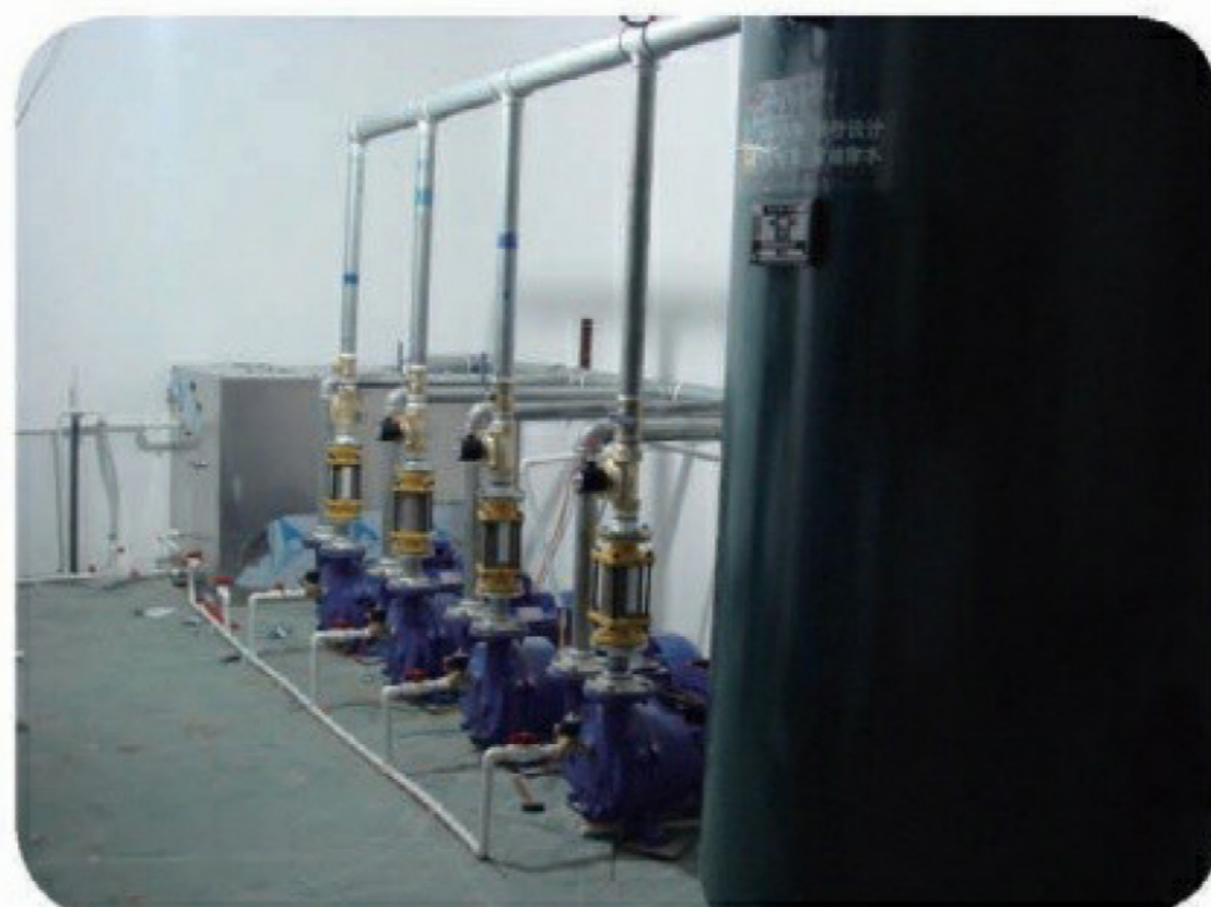
医疗负压站 Medical negative pressure station
