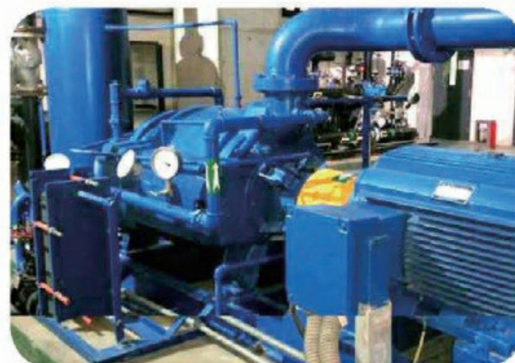
凝汽器抽真空 / Condenser Vacuum System
