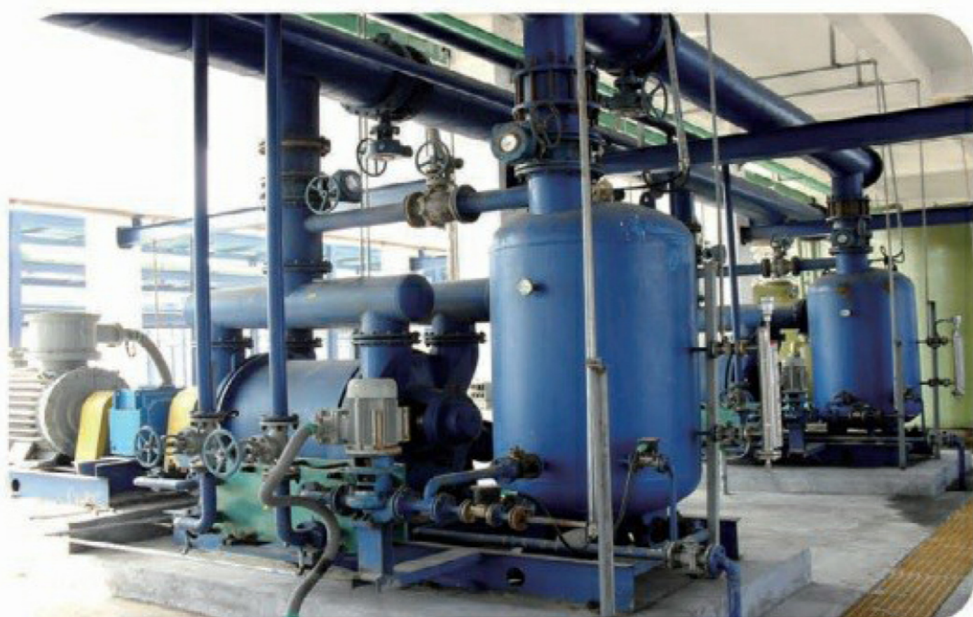
氢气乙炔压缩 Hydrogen and acetylene compression
